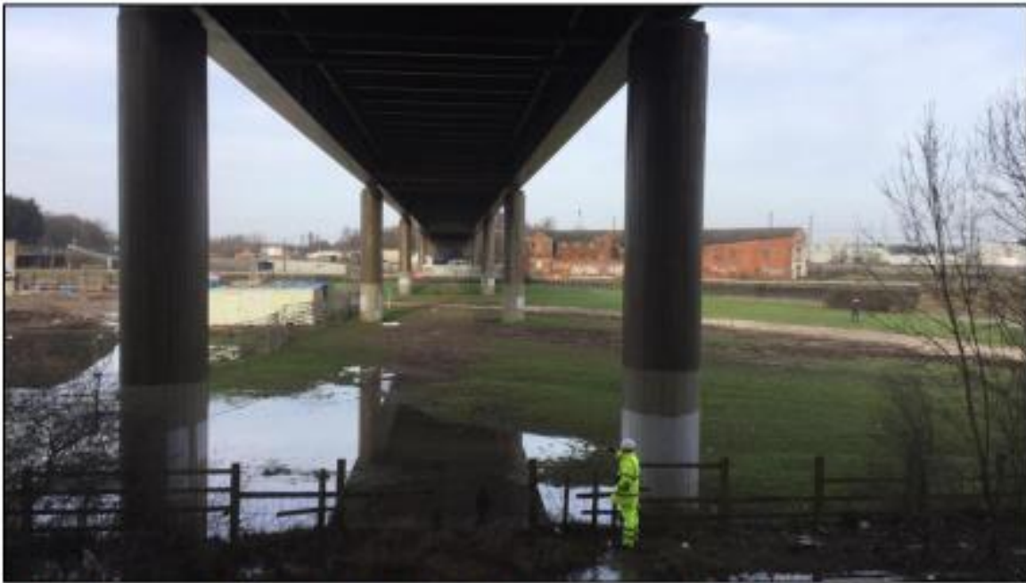
Figure 18 - Beneath Nether Lock viaduct over River Trent / East Coast Main Line looking north.
