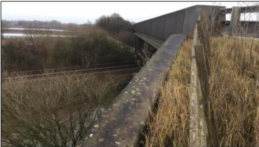
Figure 9 – A46 bridge over Nottingham to Lincoln railway line, Bridge NOB1/53A looking north.
