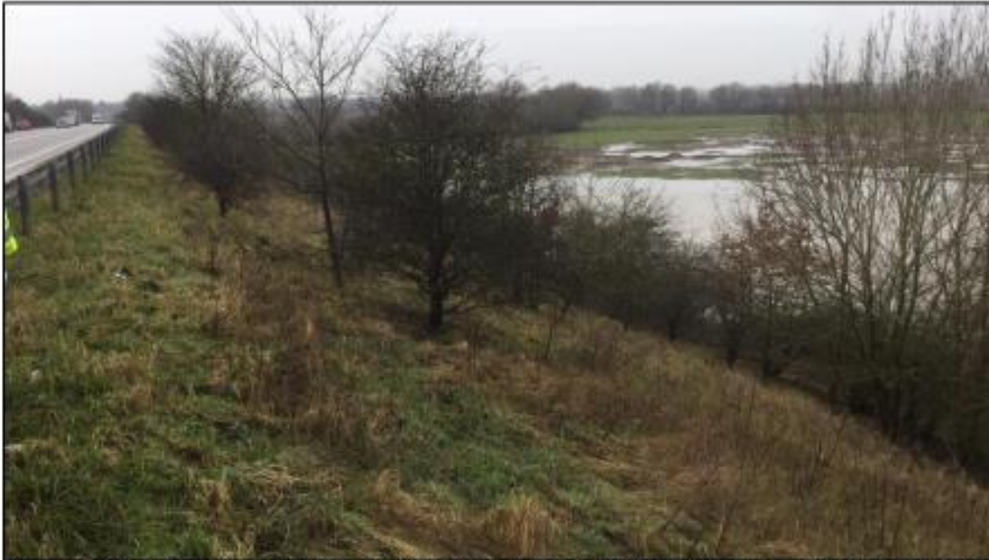
Figure 8 – General earthwork overview, looking south, between River Trent viaduct and Nottingham to Lincoln railway viaduct. Note flooded fields.
