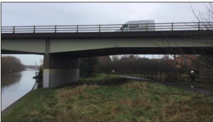
Figure 3 – Looking east, access beneath viaduct over River Trent at southern end of scheme.
